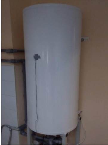
FIGURE 2: Electric heater (heat source)
