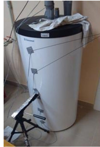
FIGURE 3: Examined hot water heater
