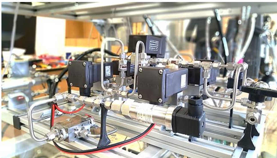
FIGURE 2: Photo of the hydrogen circuit
